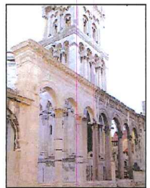
Roman Diocleziano Emperor temple (III rd century after Christ) Split (Croatia) restoration and consolidation started in the year 2005 (continuing). SPART® Products & Technologies
