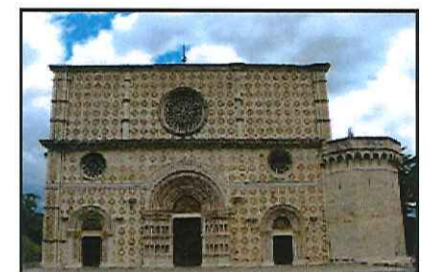
Main façade of Basilica S. Maria in Collemaggio - L'Aquila - restored and consolidated with LIME INJECTION 9000 in the year 2005 resisted to the earthquake in the year 2009! SPART® Products & Technologies
