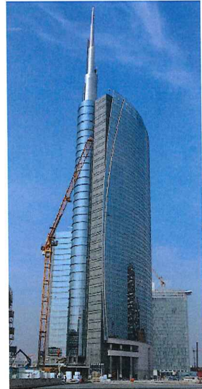
Milano Porta Nuova Garibaldi - Skyscraper Hines =231 m. INNOVATIVE CONCRETE TECHNOLOGIES! Reinforced concrete structure and columns Projected and realized with self compacting, rheodynamic concrete Rck 85 MPa pumpable up to 160 meters, workability time of 180 minutes, FIRE RESISTANT!
